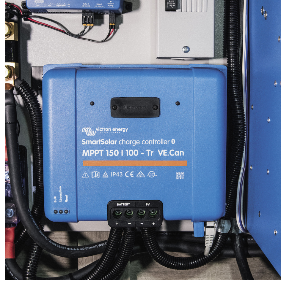
100 amp Victron MPPT Solar Charge Controller
