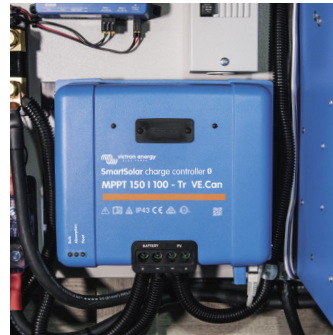
100 amp Victron MPPT Solar Charge Controller
