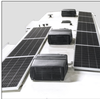
(10) 200W solar panels = 2,000 Watts of solar power
